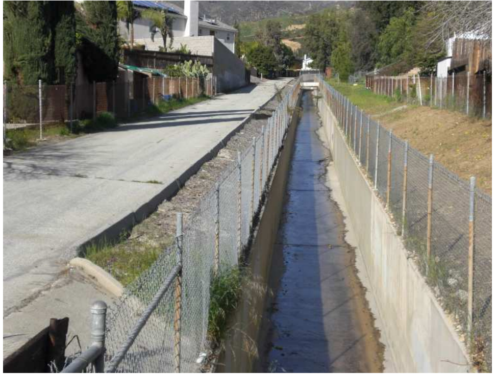
May Canyon Creek Channel at Egbert St. (upstream). Concreted portion runs from May Canyon Debris Basin for approximately 1,950 feet before it goes underground for 7,100 feet. The channel daylights right before discharging to Pacoima Wash.
