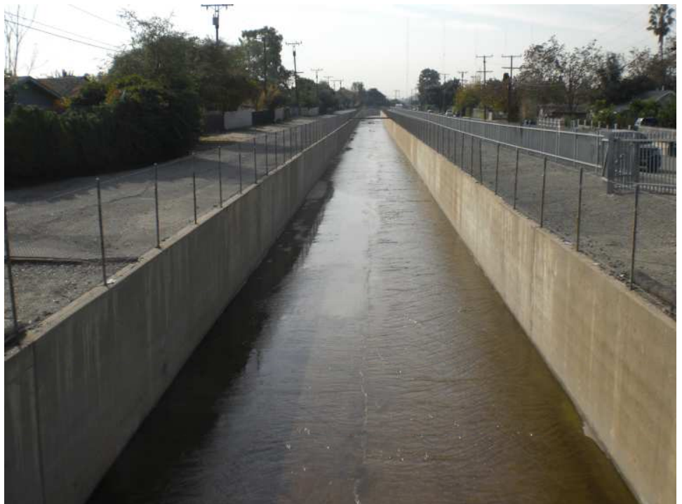
Sawpit Wash at Shroed St. (facing downstream). The channel begins at Sawpit Debris Basin and drains into Peck Road Park Lake.
