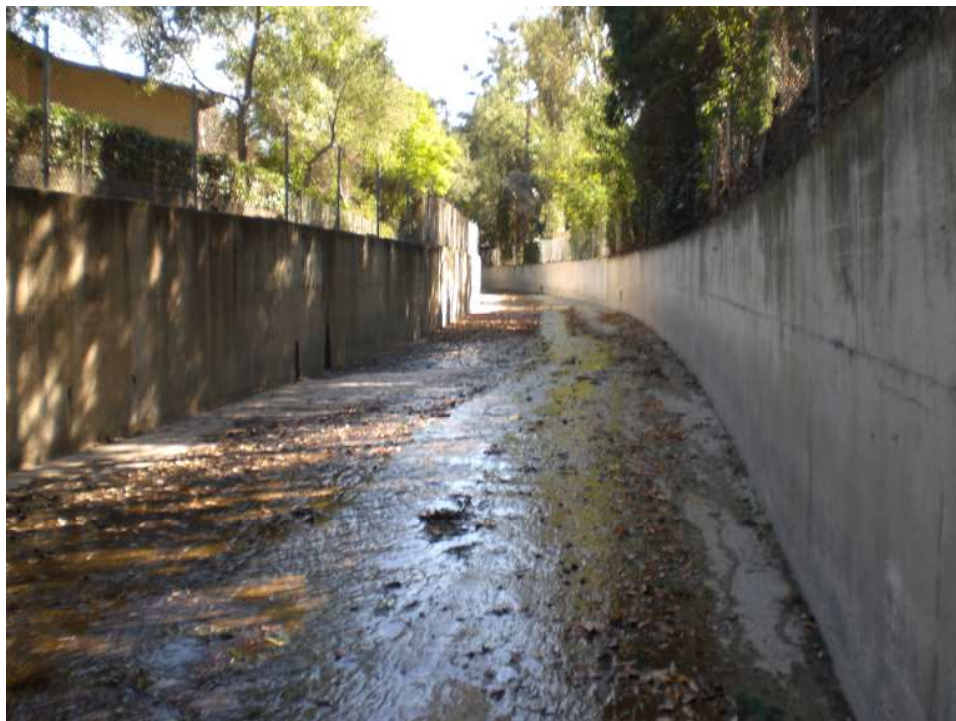
Verdugo Wash Reach 2 at uppermost concrete portion (facing downstream; photo taken inside of the channel accessed via a maintenance ramp) before the channel goes underground near the 210 freeway. The channel drains to Verdugo Debris Basin and continue to drain downstream to Reach 1 at Canada Blvd. near Verdugo Blvd. and Town St.
