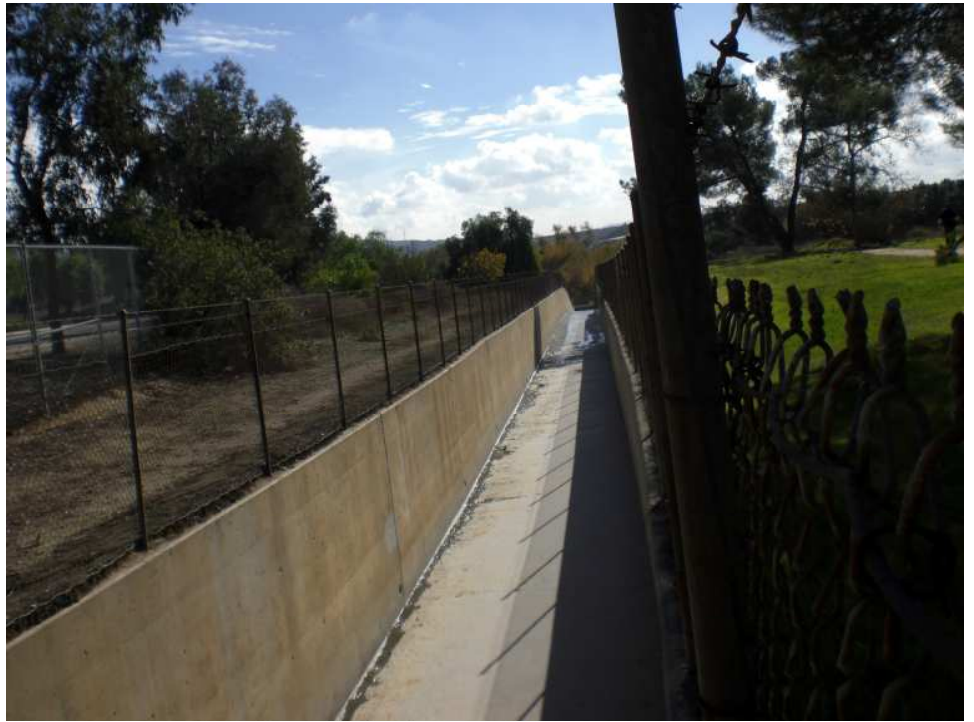
Lopez Canyon Channel at Stonehurst Ave. (downstream; Hanson Dam downstream). Hanson Dam Park on the right of the channel fence. The channel starts from Lopez Canyon Debris Basin and drains to Hanson Dam.
