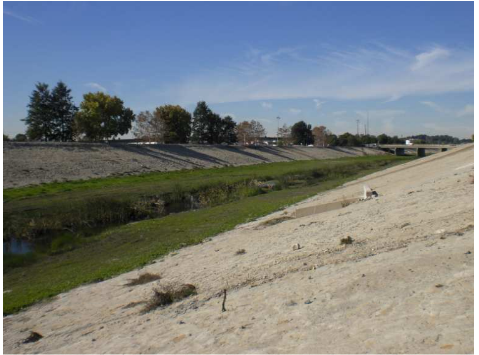
Compton Creek just upstream of its confluence with LA River Reach 2 (upstream). The trapezoidal section begins at the 91 fwy and drains to the LA River Reach 2 (~2.5 miles).
