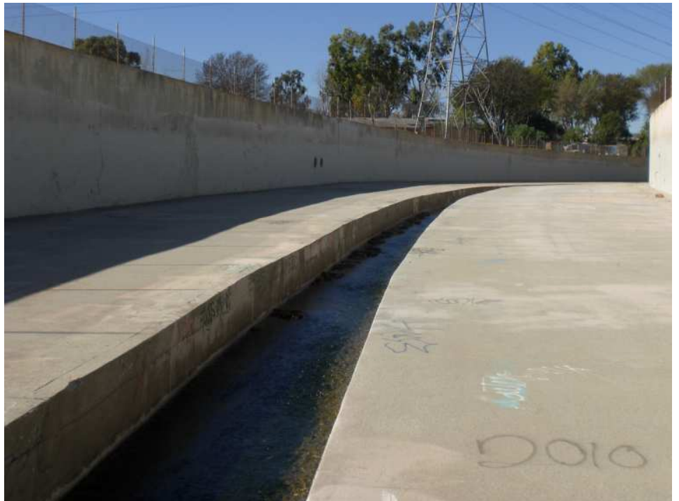
Aliso Canyon Wash upstream of its confluence with LA River Reach 6 (upstream). The channel begins at Aliso Debris Basin, drains into Wilbur Debris Basin and continues into LA River Reach 6.
