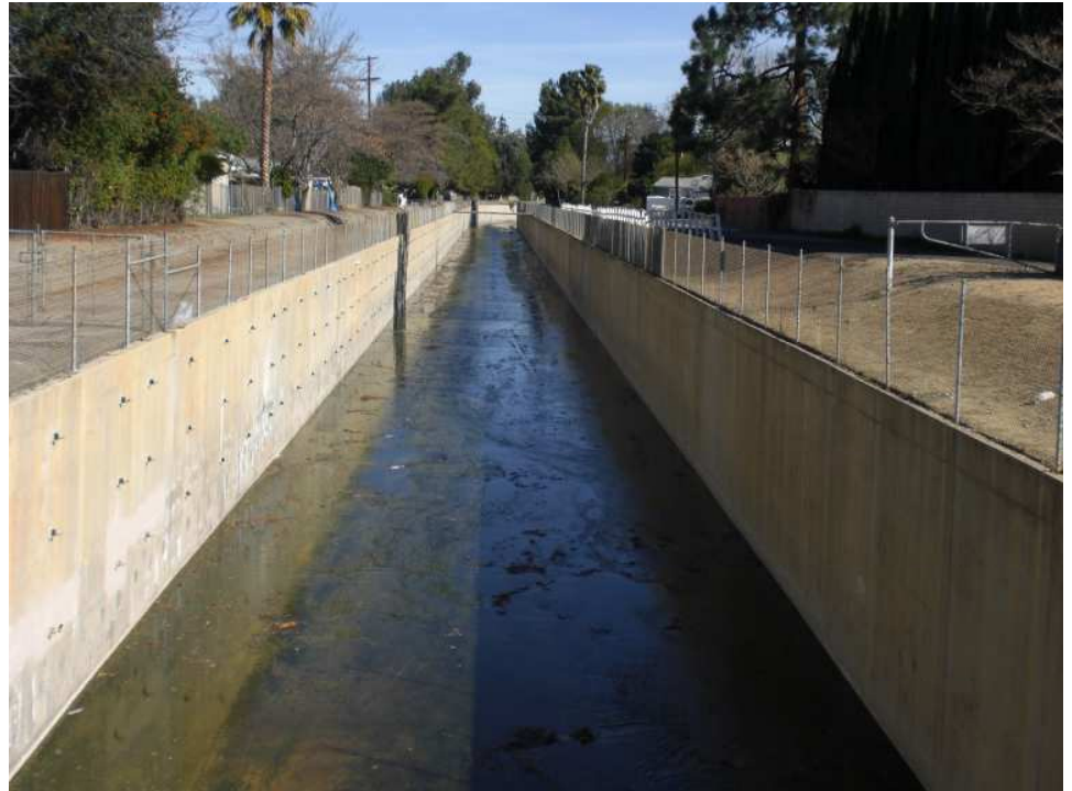
Arroyo Calabasas at Fallbrooks (downstream). The channel begins at Valley Circle Blvd. in Woodland Hills, and flows to its confluence with Bell Creek where the LA River begins.
