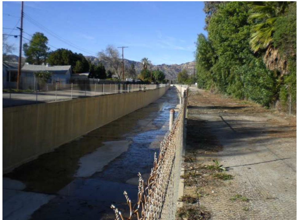
Dayton Canyon Creek (Chatsworth Creek) at Saticoy (upstream). Tributary to Bell Creek. Of the 1.3 mile stretch before its confluence with Chatsworth Creek, 0.5 miles is underground.
