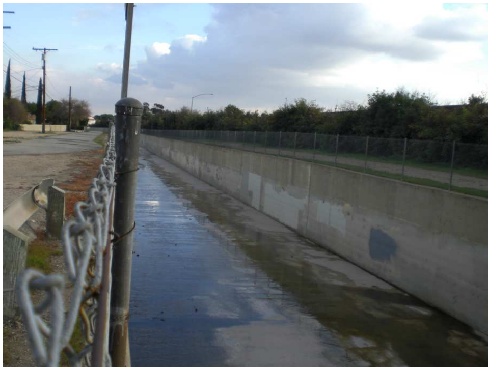
Burbank Western Channel at Lamar St. (downstream). The channel headwater is the confluence of La Tuna Canyon Channel and a minor channel. Burbank Western Channel drains to the upstream boundary of LA River Reach 3.
