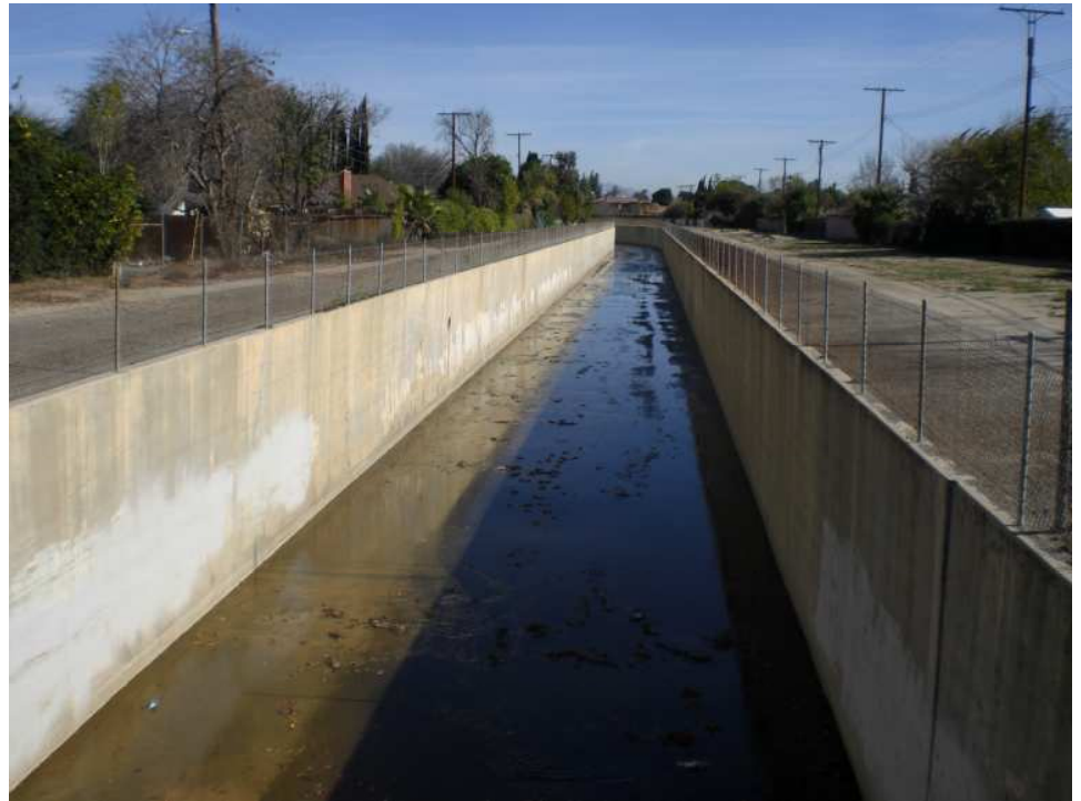
Bell Creek at Fallbrook (downstream). The concrete channel begins at Bell Creek Debris Basin and drains to LA River Reach 6.
