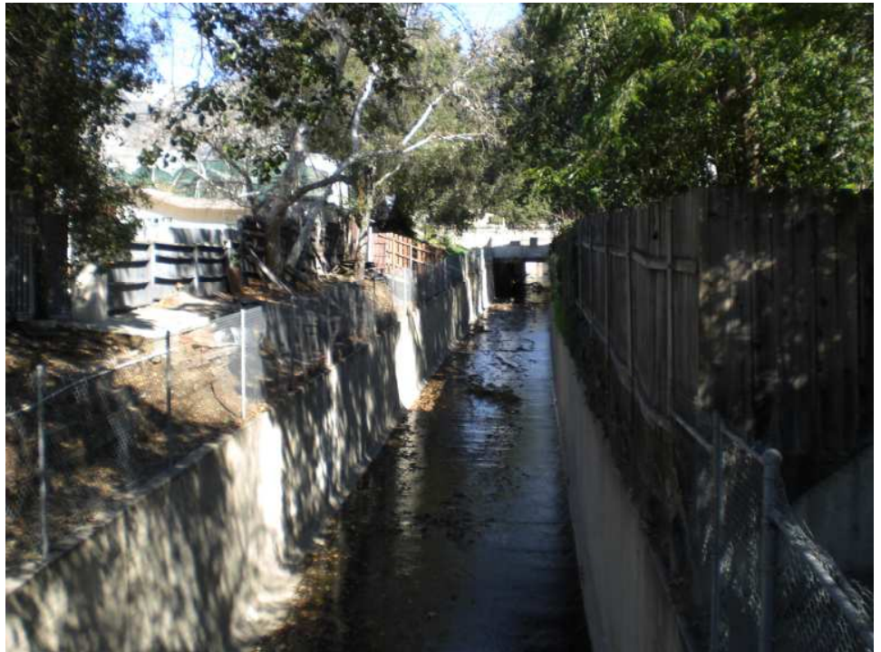
Shields Canyon Creek Channel at Miller Ave. (upstream). Concreted portion of the channel begins from Shields Canyon Debris Basin to Eagle Debris Basin. The channel continues to Verdugo Wash below Eagle Debris Basin.
