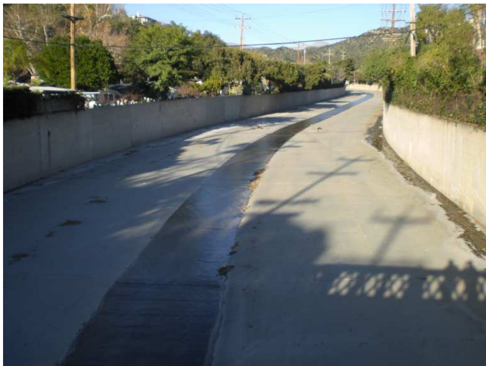
Verdugo Wash Reach 1 at Mountain St. (upstream). The channel picks up the flow from Reach 2 at Canada Blvd. near Verdugo Blvd. and Town St. and drains into LA River Reach 3.
