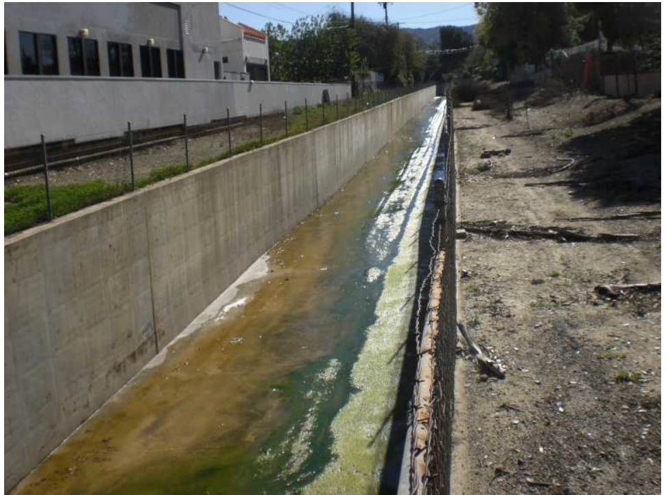
Caballero Creek at Ventura Blvd. (downstream). The concrete channel begins at Rosita St. in Tarzana and drains to LA River Reach 6.
