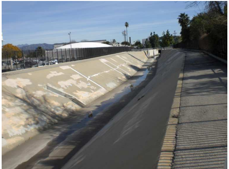
Pacoima Wash at Saticoy (downstream). The channel begins downstream of Lopez Flood Control Basin and goes underground for 3.5 miles before it reaches LA River Reach 4.
