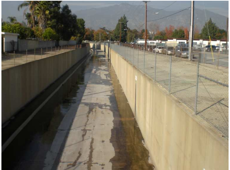
Arcadia Wash at Duarte Ave. (upstream). Underground drain receiving flow from Auburn and Bailey Debris Basins daylights at approximately 6,500 ft south (beginning of Arcadia Wash). Arcadia Wash drains to Rio Hondo Reach 3.
