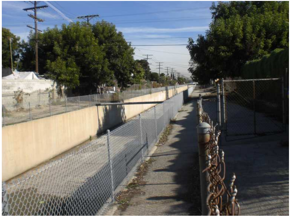
Compton Creek at Clovis (upstream). The channel daylightes at Main Street between 107 th and 108 Streets and continues (~6 miles) until the 91 fwy where rectangular shape transitions to trapezoidal.
