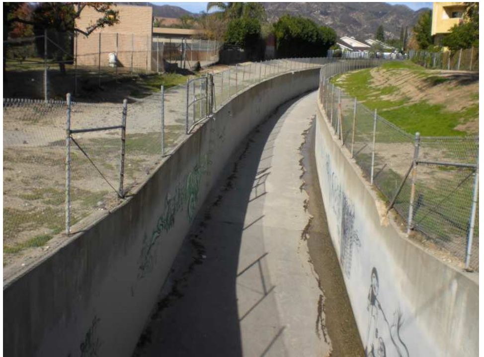
Wilson Canyon Creek at Newton St. (upstream). Concreted portion runs from Wilson Canyon Debris Basin for 7,500 feet before it goes underground for 8,000 feet. The drain daylightes right before the confluence with Pacoima Wash.
