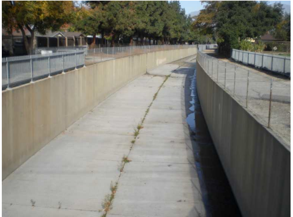
Santa Anita Wash at Liveoak St. (upstream). The channel begins at Santa Anita Dam and drains to Peck Road Park Lake. The rectangular channel transitions to a trapezoidal channel less than half a mile before draining into the lake.
