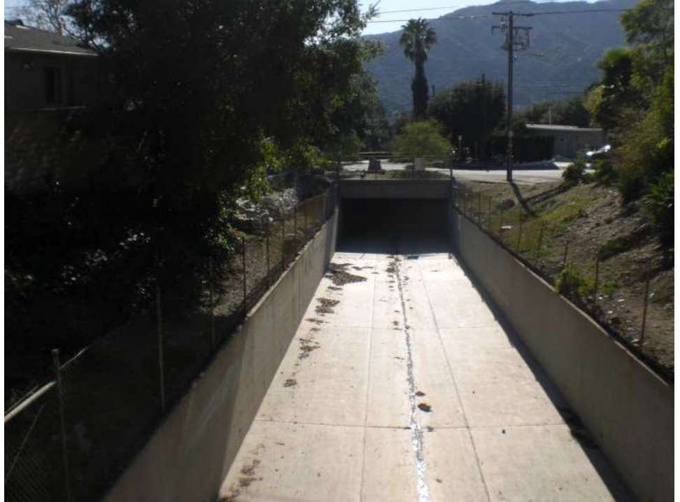
Pickens Canyon Creek at Mayfield Ave. (downstream). Concreted portion begins at Pickens Canyon Debris Basin and drains into Verdugo Wash Reach 2.
