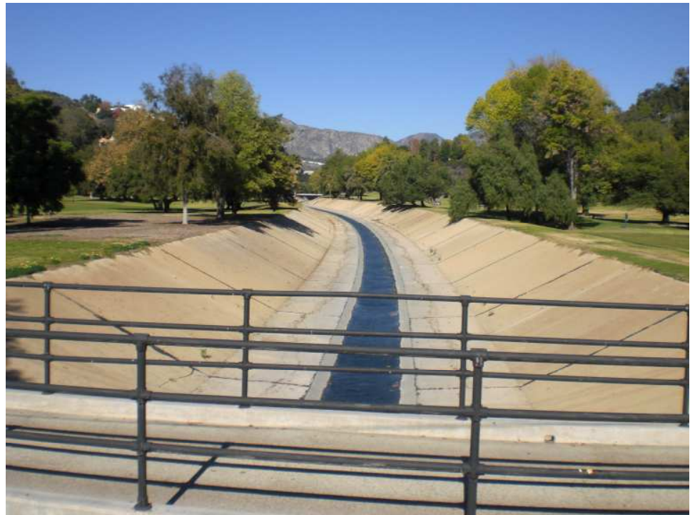
Arroyo Seco Reach 2 at the Brookside Golf Course (upstream). The channel begins below Devils Gate Dam and flow to Arroyo Seco Reach 1 at Holly St. Of the 2.3 mile reach, the downstream 0.5 miles is a rectangular channel.
